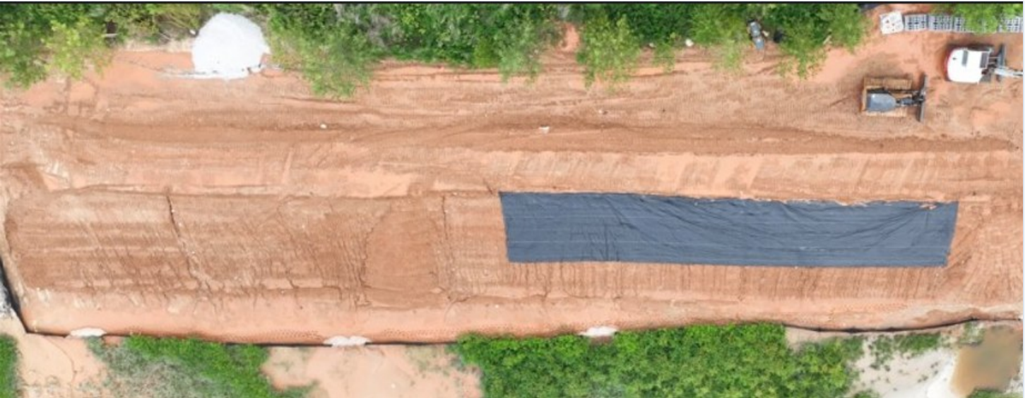
Fig. 9 — Graded haul corridor; surface condition and standing water after rain.
